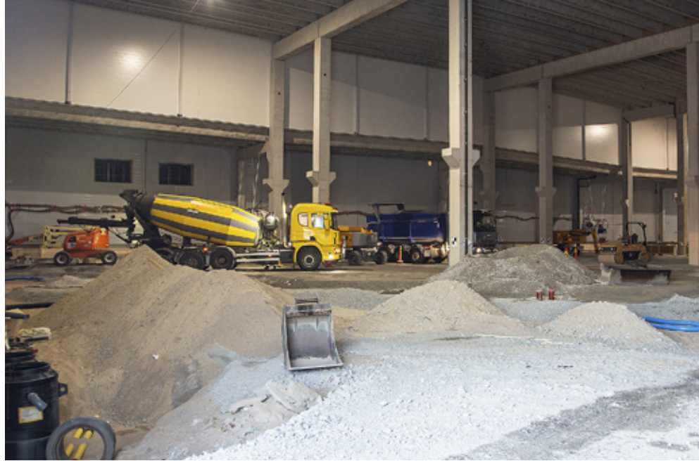
The number of construction workers at the transmission plant has averaged around 20, but the number has varied a lot according to the construction phase.
